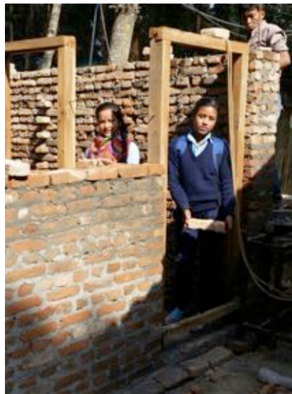
In Kavre, Little Sisters worked with community members to build a new school toilet.
